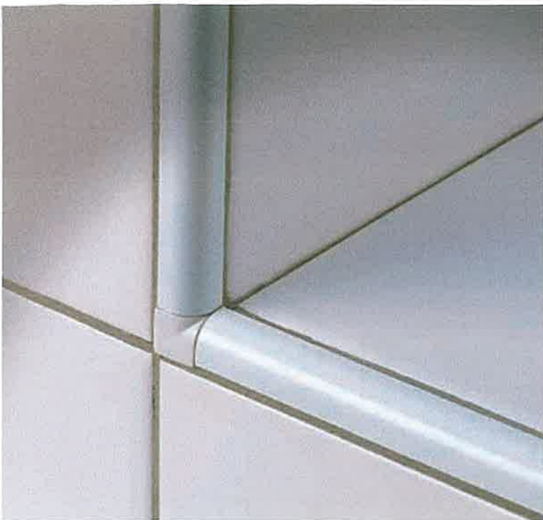
Wall section where the application of the jointing RJ capsule for the profile trim finish is evident.
